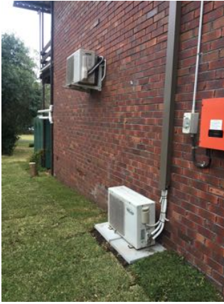
Air conditioning overflows Western side
