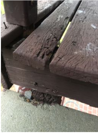
Rotting decking boards and bearer
