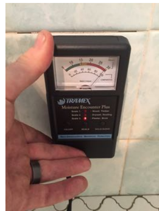
High comparative moisture reading up stairs shower recess
