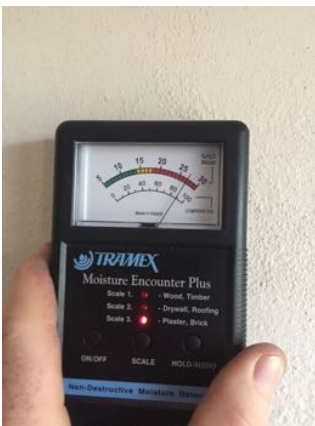
High comparative moisture reading walls of down stairs shower recess
