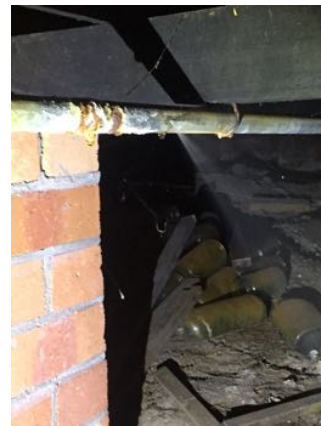
Leaking water pipe Northern area sub-floor
