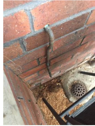
Hot water system pressure relief valve Northern side
