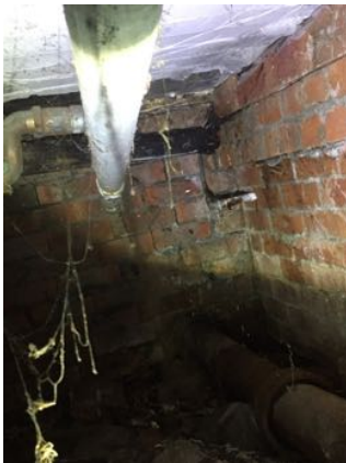
Rotting bearer Northern side under bathroom and laundry.
