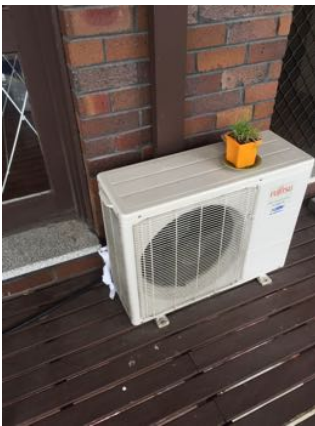
Air conditioning overflow Northern side
