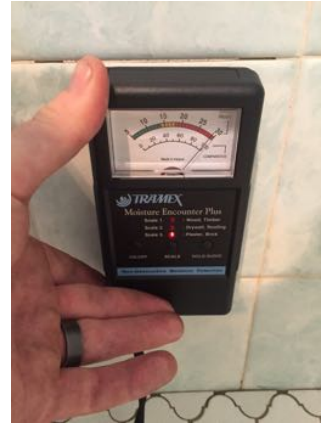
High comparative moisture readings in upstairs shower walls
