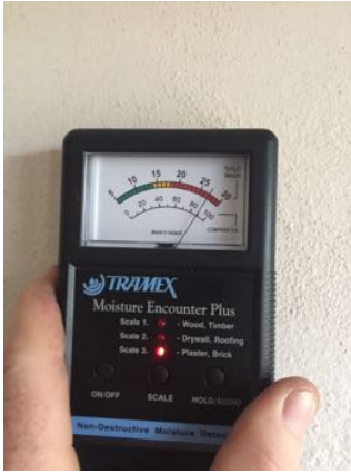
High comparative moisture readings in down stairs shower walls
